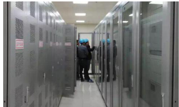
Figure 3 Control and Protection System of 220kV UPFC Project in Nanjing, China
