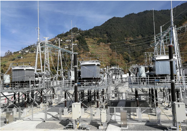
Figure 2 220kV Fixed Series Compensation Site
