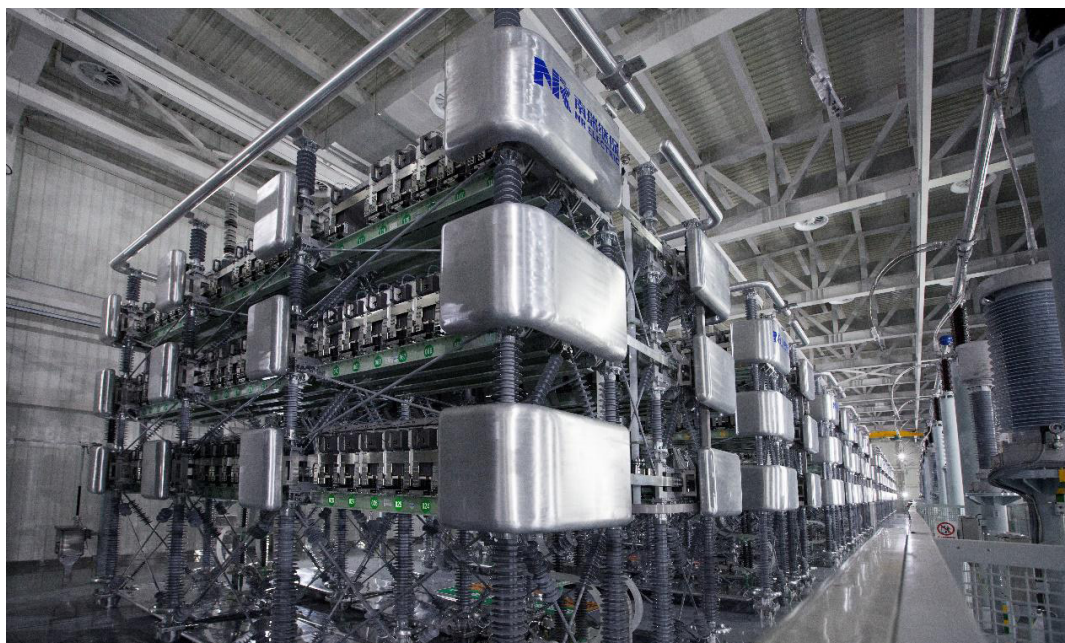
Figure 5 VSC Valve of 500kV UPFC Project in Suzhou, China
